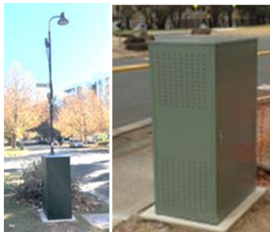
Figure 3: Carrier-provided image of required 5G cabinet required to sit beside any pole carrying 5G equipment in Elizabeth St Mall. Note that in the left hand image, the transmitter on the pole is barely visible, but the cabinet is a large piece of infrastructure, 1.3 m high, 0.5 m deep and 0.8 m wide
