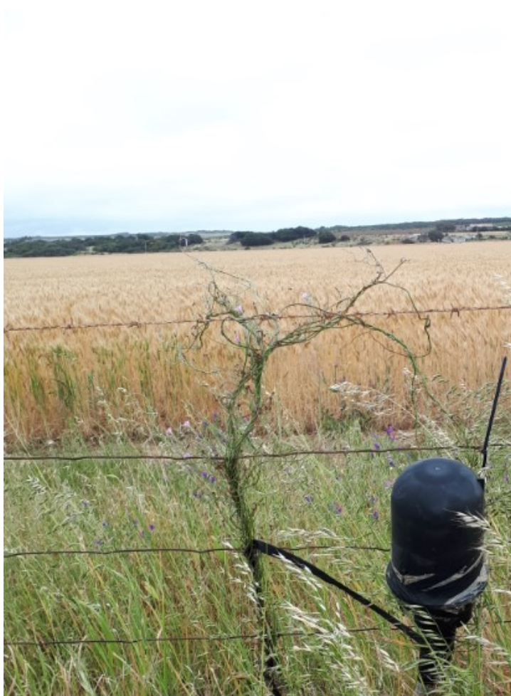
Figure 6: A telecommunications cable affixed to a farmer's fence in the road corridor.
