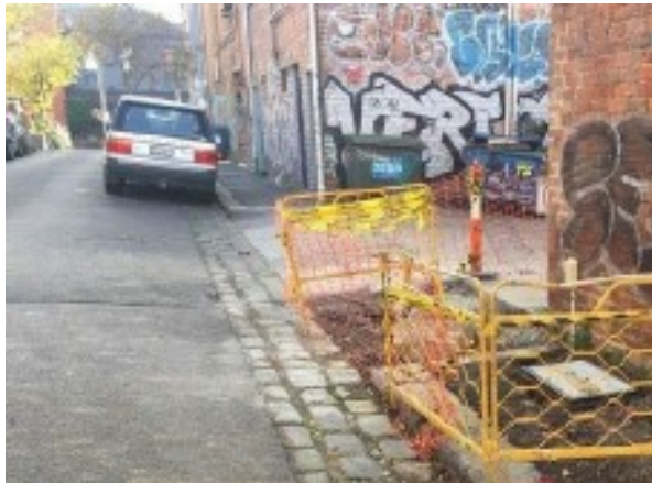
Figure 19: Site was reportedly left in this condition for a week, before crews came back to finish off the works. There was no notice regarding these works and no correct signage indication footpath is out of use.
