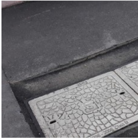
Figure 14: Pit is located at a bus stop. This reinstatement failed due to poor compaction of the subgrade layers and the top layer of asphalt. Resulting in a large lip against pit, causing a severe tripping hazard.
