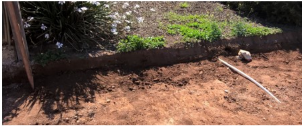
Figure 5: Telecommunications conduit installed directly beneath the footpath and not to the minimum depth required by good engineering practice in the road reserve negatively impacted footpath replacement costs and timeframes.
