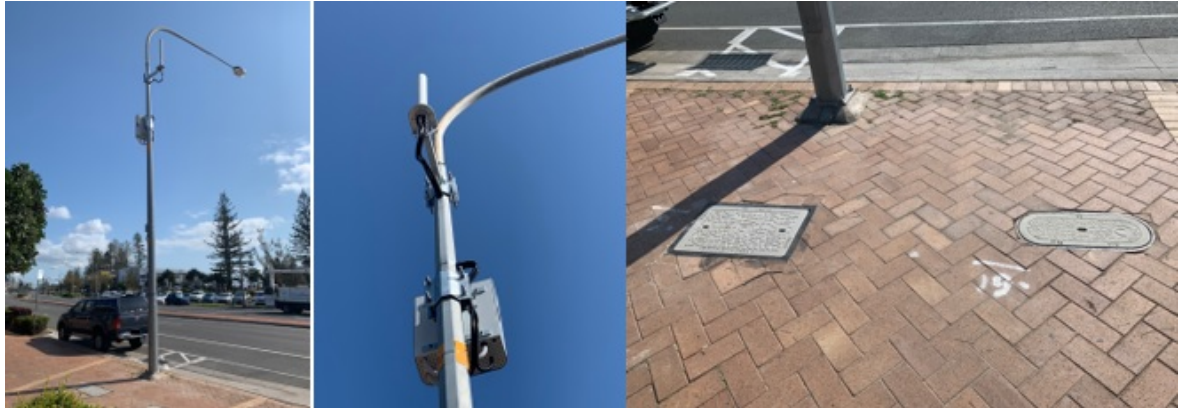
Figure 10: Example of what a below ground cabinet small-cell split installation is expected to look like in a road. Note that the streetlight pole has been drilled into (damaging the pole) to facilitate electricity and fibre connections to the installation on the pole.
