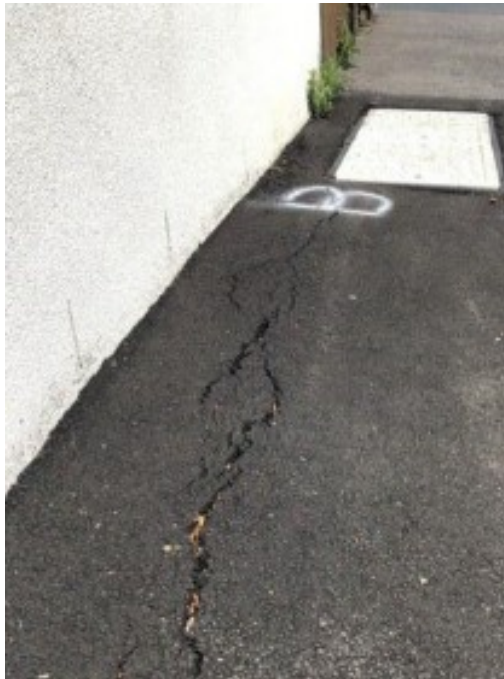
Figure 18: Reinstatement failed causing tripping hazard along footpath. Cracking along reinstatement works indication that insufficient compaction was applied throughout layers of reinstatement.
