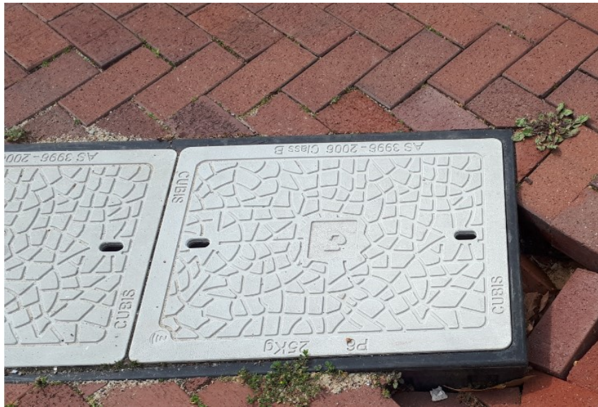
Figure 11: An example of poor reinstatement on a footpath creating a hazard for pedestrians and cyclists.
