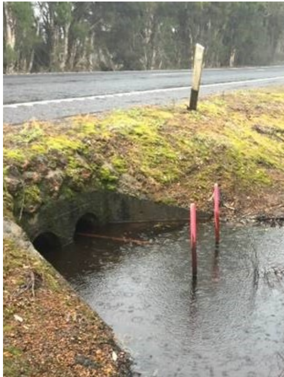
Figure 4: The orange telecommunication cable at the culvert opening has restricted debris resulting in a blocked drain. The road authority is unable to clear the culvert or undertake scheduled culvert extension works (addressing a road safety hazard) without removing the cable.
