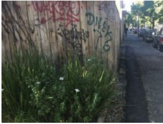
Figure 17: Trench was left in a temporary condition, in cold mix asphalt. Too much cold mix was used resulting in a hump being formed along the footpath, as well as leaving loose cold mix scattered along the footpath. This results in a slipping hazard to all pedestrians that use the footpath.
