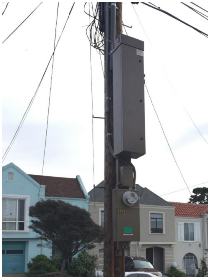
Figure 9: Example of an all in one installation (Image © Creative Commons)
