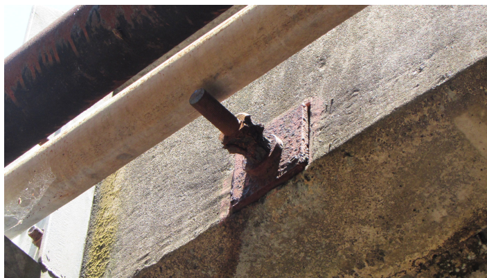
Figure 2: Telecommunication conduit resting on a transverse stressing bar of a bridge, increasing oxidization of the bar, and preventing the road authority from undertaking bridge maintenance (replacement of the bar). This bar is critical to the bridge integrity and safety.
