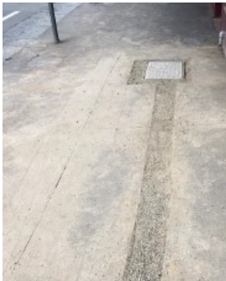
Figure 16: Footpath left in crushed rock without any compaction, it is council standard to use cold mix as a temporary reinstatement. Leaving this in crushed rock causes rocks and dirt to be spread across the footpath causing a slip and trip hazard to anyone using the footpath.
