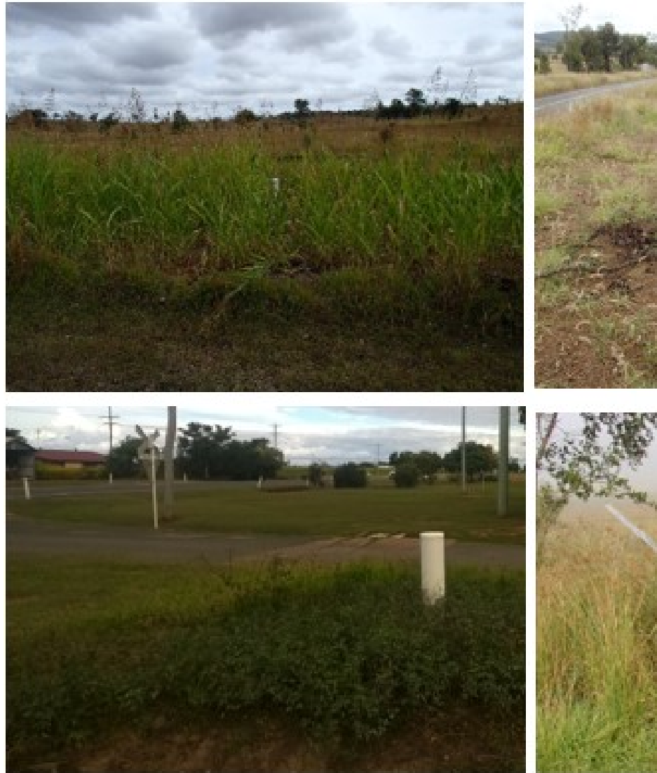
Figure 7: Elevated joints are a common problem, especially in agricultural areas. Elevated joints are usually repaired cables that are not re-buried, they often do not comply with road clear zone requirements. When road verge becomes overgrown then road authorities can impact these joints during roadside vegetation slashing and fire management.
