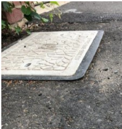
Figure 15: This reinstatement failed due to poor compaction of the subgrade layers and the top layer of asphalt. Resulting in a large lip against pit, causing a severe tripping hazard.
