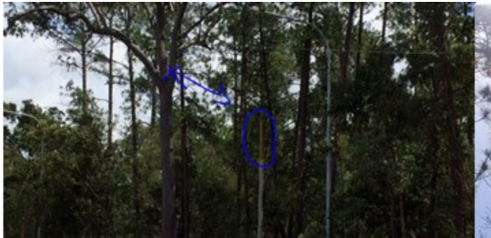
Figure 3: Overhead telecommunications cable installed by a carrier's contractor into a tree. The cross indicates where the cable was attached to the tree and the arrow shows the extended pole that was modified for additional attachment.
