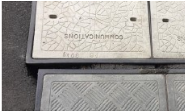
Figure 20: Placement of pits are too close to one another. Not allowing correct compaction to be made between pits. Resulting subgrade failure.
