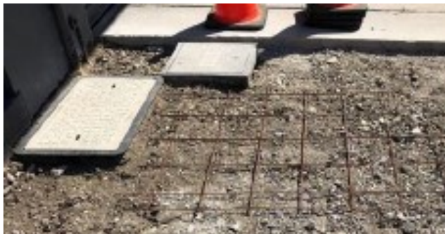
Figures 13: This was a site that was caught during the works and was noted that; Bedding layer was not compacted, insufficient amount of mesh used, no bar chairs used and no expansion joint material was used. Without these elements the reinstatement will fail in due time, and become a hazard.
