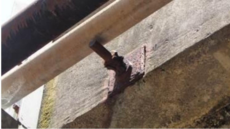
Figure E: Telecommunication conduit resting on a transverse stressing bar, increasing oxidization of the bar, and preventing the road authority from undertaking maintenance (replacement of the bar). This bar is critical to bridge integrity and safety.
