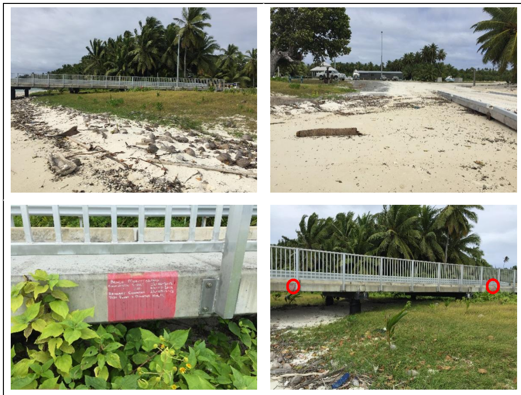
Figure 19 Clockwise from top left: Accreted area at jetty abutment; old ramp versus new ramp; old survey marks (2013); location of old survey marks on jetty
