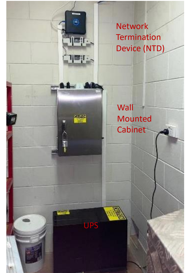
Large site set-up showing UPS and cabinet
