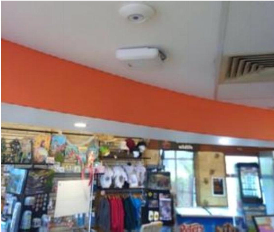
Wireless Access Point (circular feature at top centre of photo)
