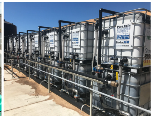
Stand alone filter system to filter metals from industrial sites. Photo by Ryan Holmann, Stormwater Biochar; filters by BioLogical Carbon
