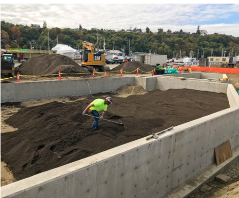
Stormwater vault. Photo by Sarah Burch
