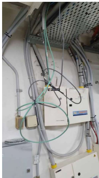
Figure 2: Cabling not fixed properly in MDF room
