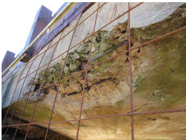
Figure 24: Bridge deck concrete cancer
