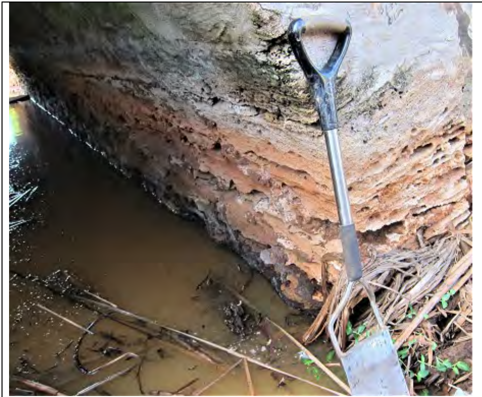
Figure 2. Pier street bridge showing exposed corrosion / dissolution of cement mortar and calcarenite used in the construction of the Pier street bridge – photograph taken in February 2020 during the drought/ dry period.
