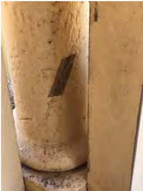
Figure 6 Column defect (bottom)
