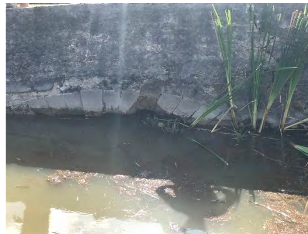
Plate 5 Detail of western arch of the Bounty Street Bridge prior to dewatering. AECOM 2020.
