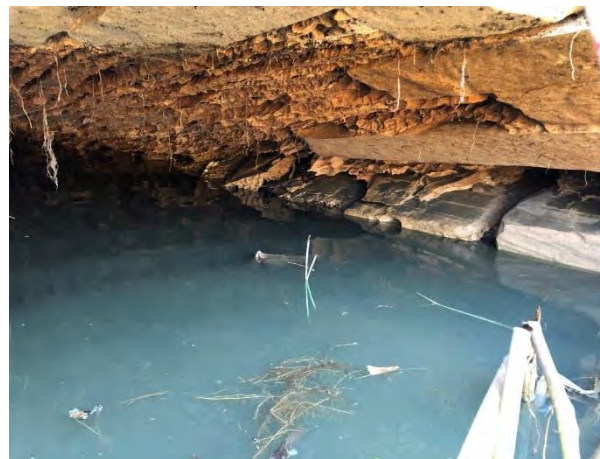
Plate 9 Soffit erosion near western arch. AECOM, 2020.
