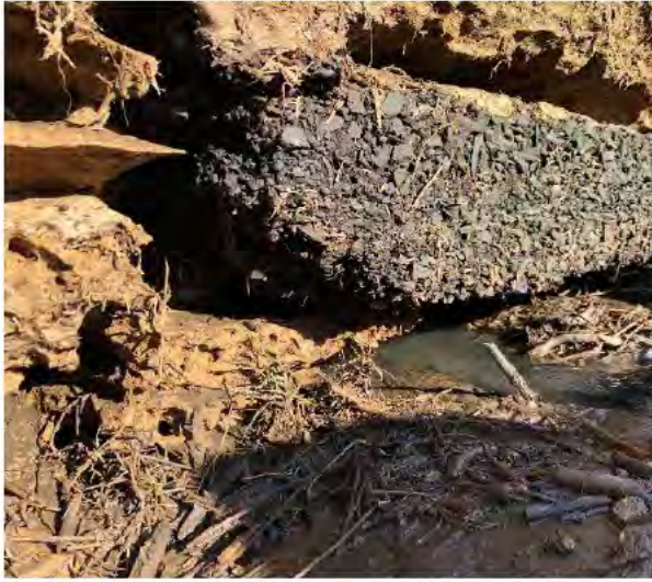
Figure 8 Stone Abutment and Lintel Erosion
