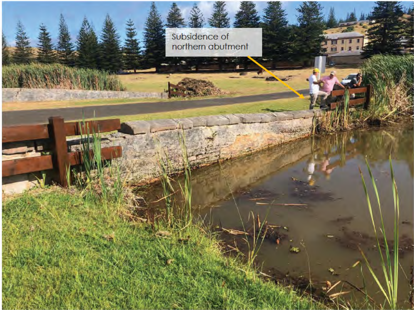
Photo 1 – 28/1/2020 – View of the Bounty Street Bridge, looking NW. The subsidence of the northern abutment can be seen clearly.
