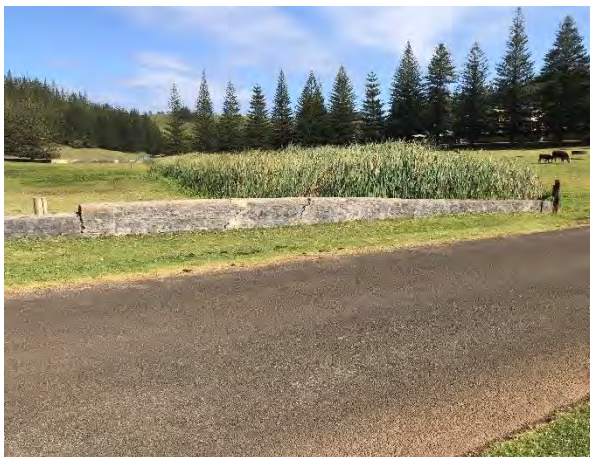
Plate 4 View west showing western wall of the Bounty Street Bridge. Note crack in parapet wall. AECOM 2020.
