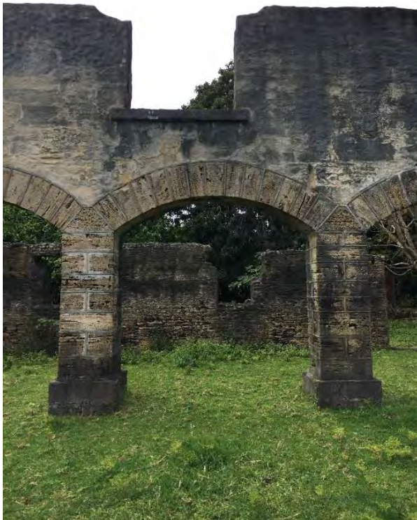
Figure 11 Arch and window misalignment
