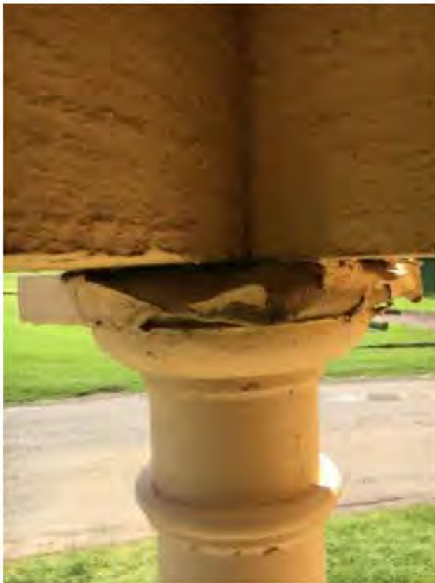
Figure 7 Eroded capping stone
