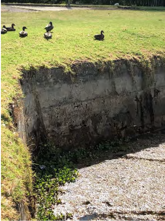
Figure 18 Eroded dam lining
