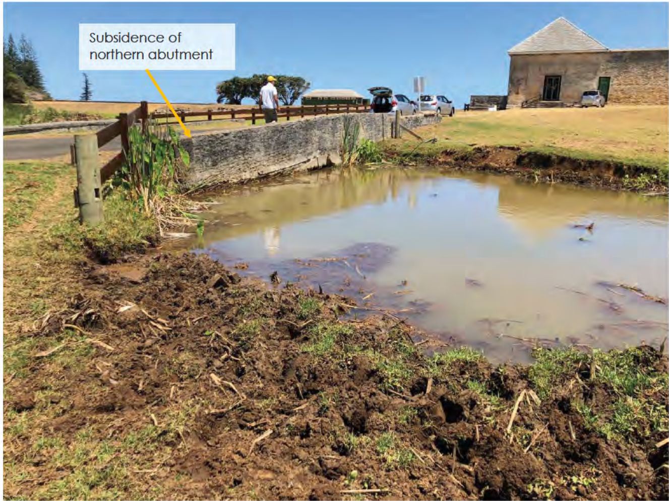
Photo 2 – 28/1/2020 – View of the Bounty Street Bridge, looking SE. The subsidence of the northern abutment can be seen clearly.
