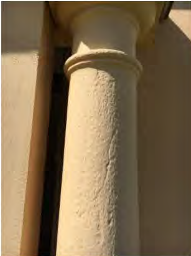
Figure 5 Column defect (top)
