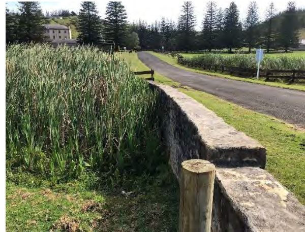
Plate 3 View north along the western side of the Bounty Street Bridge. Note coping stones are missing.
