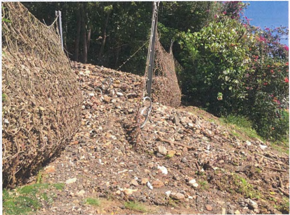
Boat Club landslide debris captured at fence line
