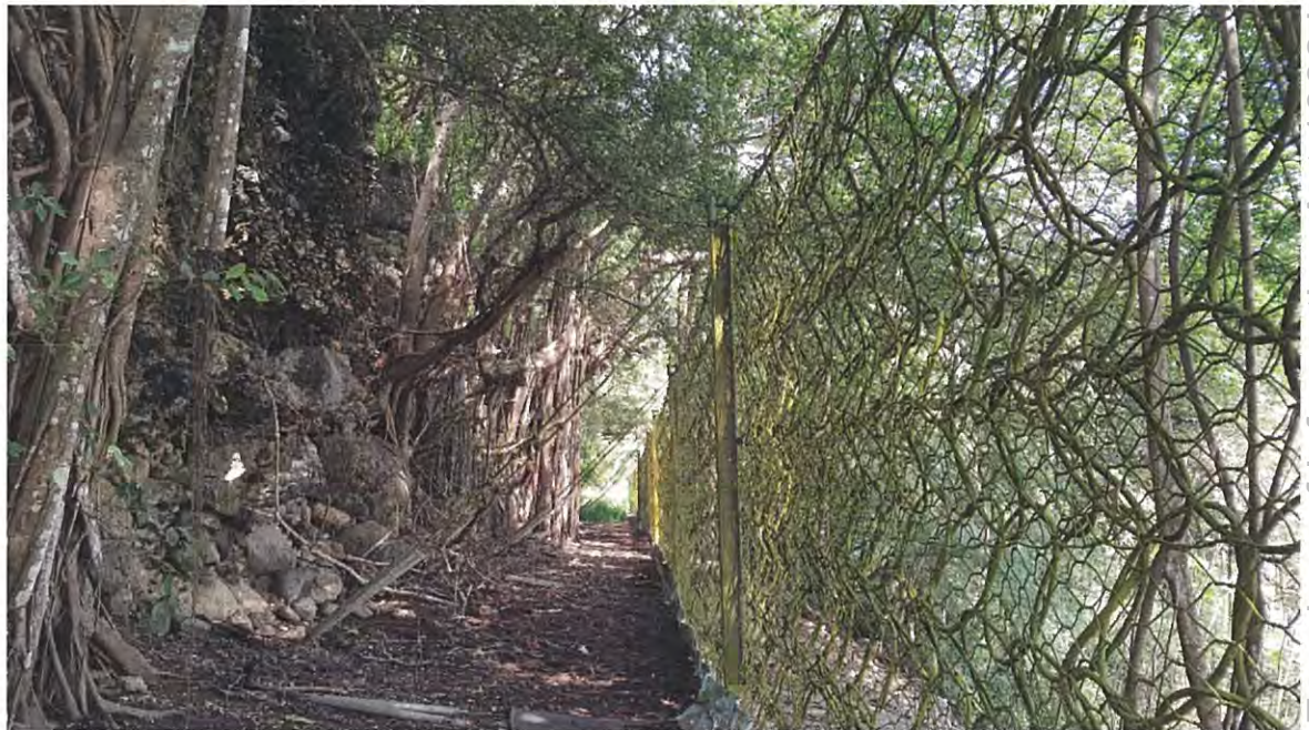
Figure 7. Former Railway Line Area and Cutting (left). 'Christmas Island Club' Rockfall Barrier on Right.
