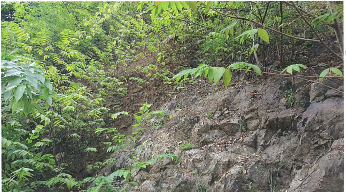
Figure 6. Soil Profile (left) Exposed in Flank of Basketball Court' landslide
