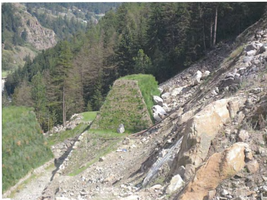
Figure 16. Green Terramesh® embankments providing rockfall protection to road, Aosta Valley, Italy (Photo courtesy of Maccaferri Pty Ltd / Geofabrics).
