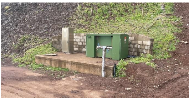
PHOTOGRAPH 2-7 DESALINISATION PLANT WATER POINT (ERM 2025)
