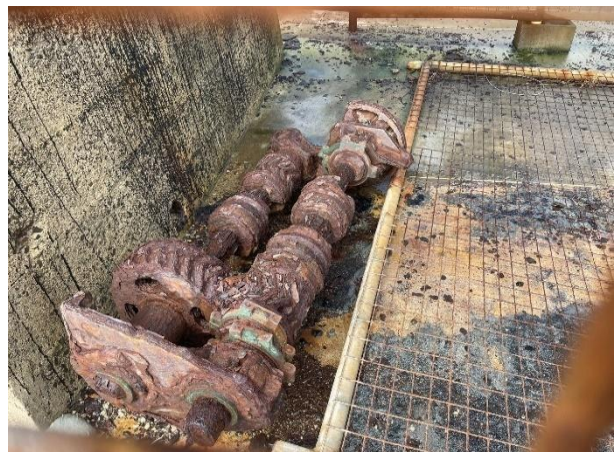
PHOTOGRAPH 2-16 UNDER THE BOILER WITH FLAKES FROM SURFACE (ERM 2025)
