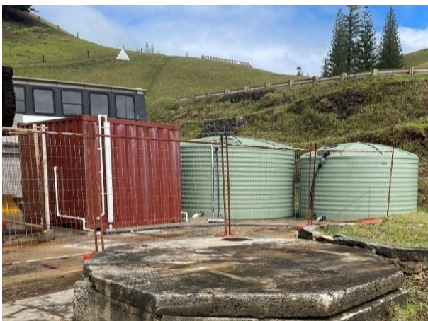
PHOTOGRAPH 2-11 UPPER PLATFORM WITH DESALINATION PLANT (ERM 2025)
