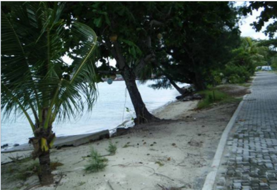
Figure 12: Jalan Pantai on Home Island prior to seawall construction (2) indicating the low elevation of the road and narrow foreshore, 29 May 2009 (DoT, 2010)
