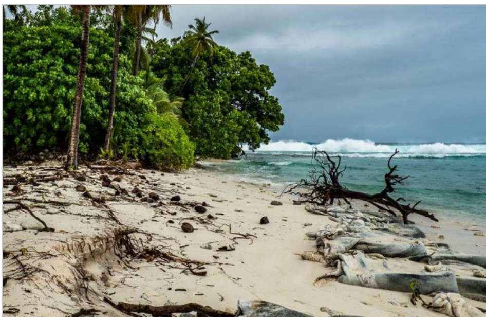
Figure 14: Trannies Beach erosion and failure of seawall following July 2018 event (RHDHV, 2021a – source: Karen Willshaw)
