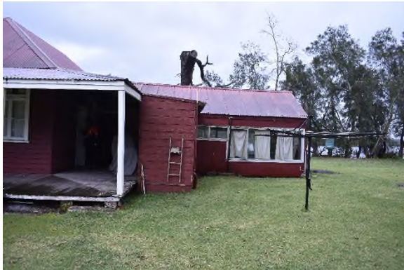
Figure 105 Northern end of eastern elevation, showing cardroom on lean and in poor condition.
