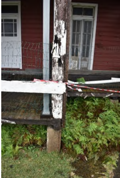
Figure 135 Decaying verandah post on western elevation.
