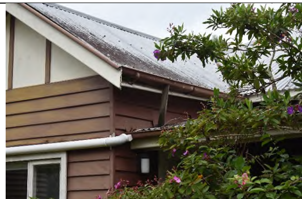
Figure 75 Ad hoc support for a gutter on Ardath Cottage.
