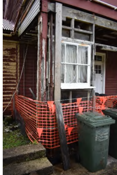
Figure 136 Location of removed annexe on eastern verandah, with timber in poor condition.
