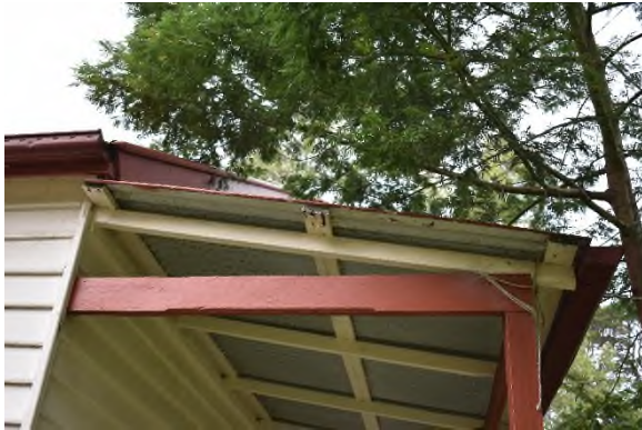
Figure 96 Verandah sheeting with no gutter.
