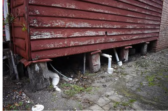
Figure 140 Timber pilings in poor condition.
