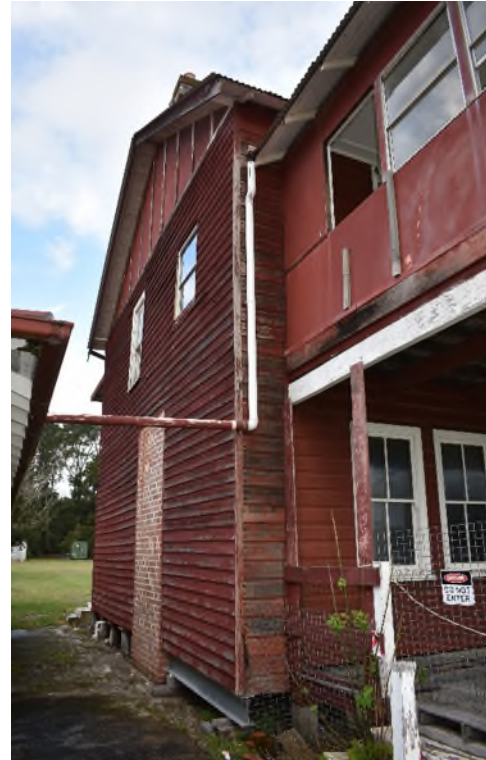
Figure 144 Northern elevation side of building, with unsympathetic services installation and verandah enclosure on upper level.
