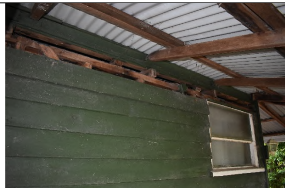
Figure 54 Missing external weatherboards.
