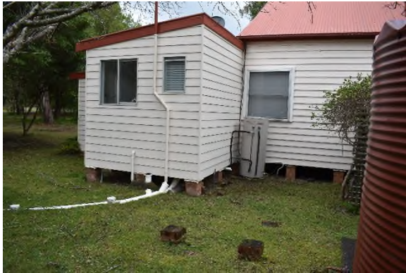
Figure 90 Northern elevation showing unsympathetic installation of services.
