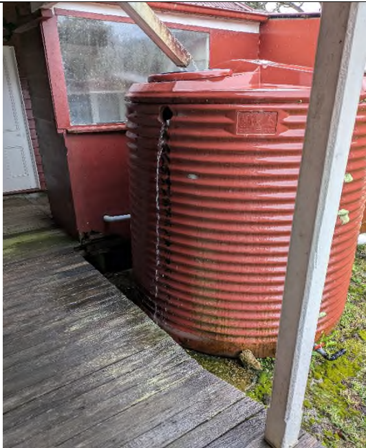
Figure 113 Water tank overflowing directly to the verandah decking, posts and building foundation.
