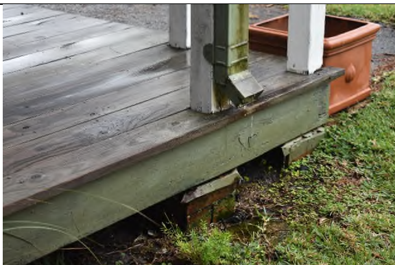
Figure 53 Downpipes draining directly to soil and building foundations.
