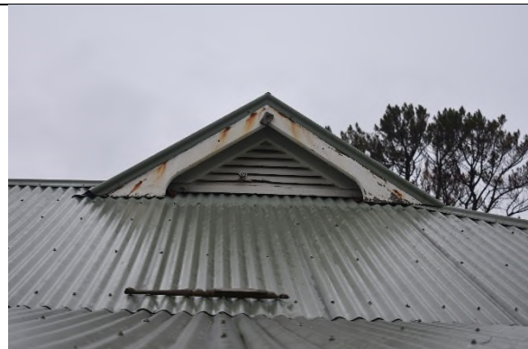
Figure 40 Non-original decorative finial has fallen from the roof.
