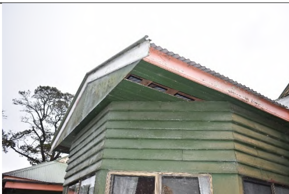
Figure 47 Missing soffit board on southern elevation.
