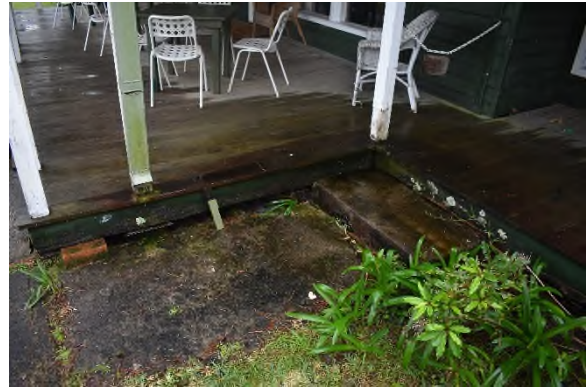
Figure 44 Example of rain around verandah boards and moss growth.
