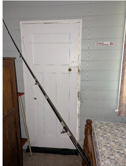
Figure 112 Internal door to western verandah. Note spiderwebs and door does not hang flush.
