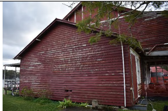
Figure 134 Southern elevation, with gaps in weatherboard on lower part of wall.
