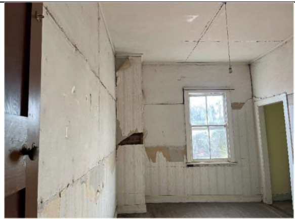
Figure 150 Upper floor interior, 2024. (Source: ACOR Block 14 Building Audit Report)
