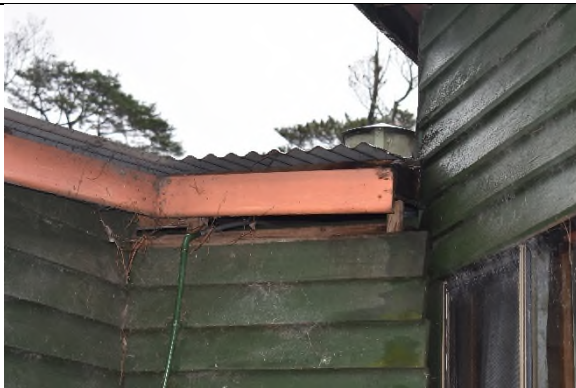
Figure 45 Loose fascia on southern elevation.
