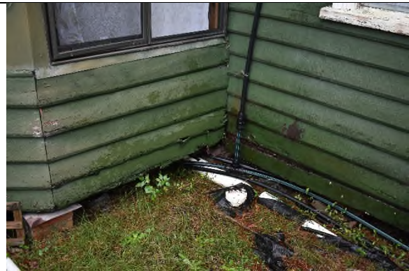
Figure 46 Weatherboards in poor condition on southern elevation.
