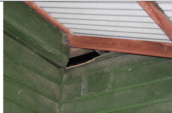
Figure 52 Missing external weatherboard.
