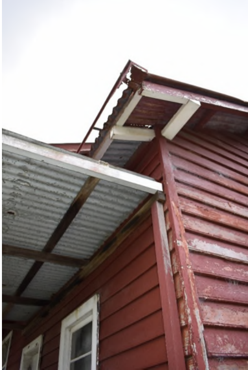
Figure 143 Rusted, non-functional gutter.
