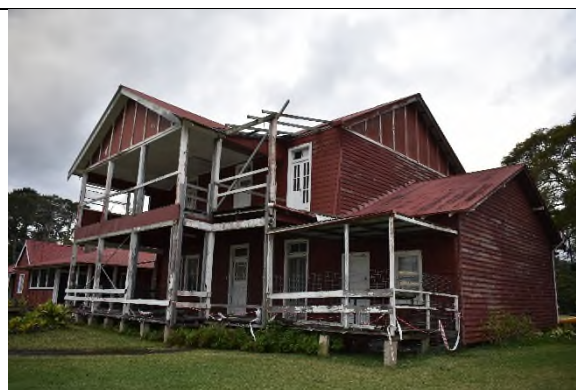
Figure 130 Christian's Minde southwestern corner. Note verandah framing on upper level where roof sheeting has blown off.
