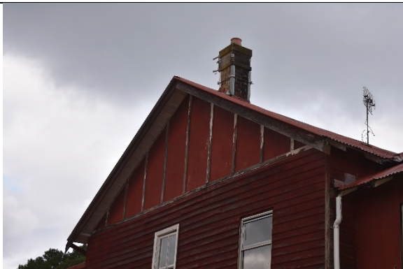
Figure 107 Detail of southern end, with chimney secured by metal straps and gable end cladding in poor condition.
