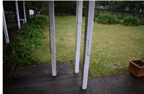
Figure 50 Previous repairs to verandah posts.
