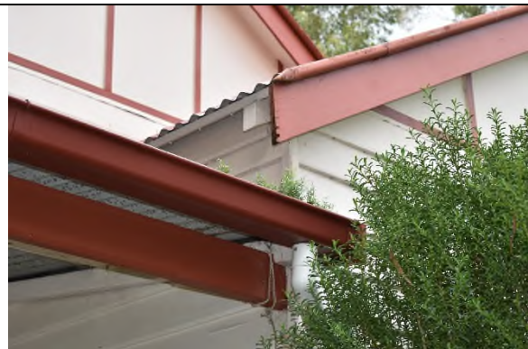
Figure 95 Vegetation growing in gutter of Pamir Cottage.
