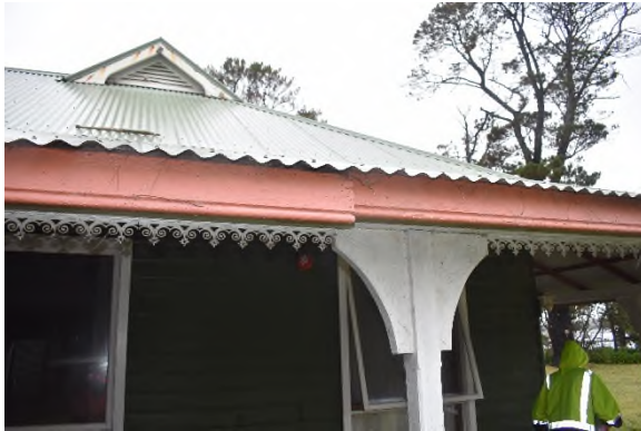
Figure 49 Misaligned fascia and plastic decorative lace work.
