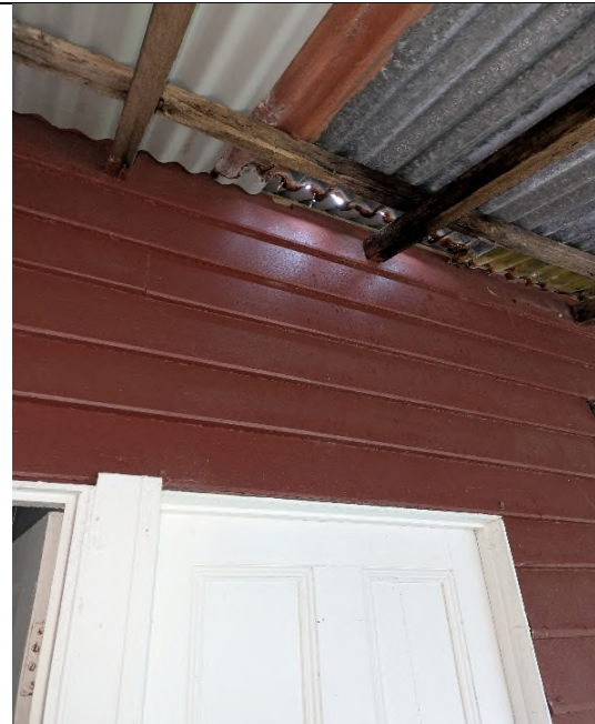
Figure 114 Hole in verandah roof sheeting.
