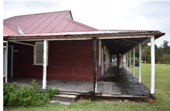
Figure 106 Northwestern corner, showing decaying verandah posts, loose gutter and verandah boards in poor condition.
