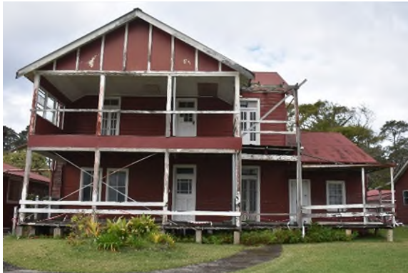
Figure 3.84 The front (western) elevation of Building CM3. Verandah with missing roof sheeting is visible on the upper floor at the right-hand corner.
