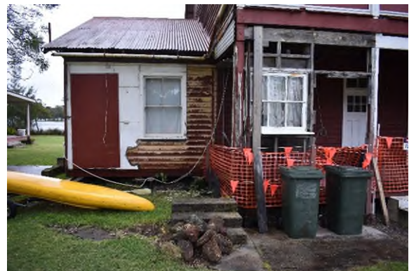
Figure 3.87 Building CM3 on the eastern (rear) elevation showing the decayed and removed fabric from the verandah and single-storey addition. The partially exposed weatherboard around the leftmost window is the location of a removed laundry annexe.
