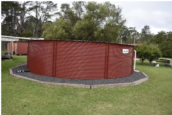
Figure 3.92 The water tank installed southwest of Building CM5.
