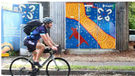
Figure 72. Community battery in Cammeray, NSW.
