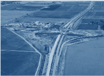
An aerial view of the Curtis Road Interchange, part of the Northern Expressway Project.
